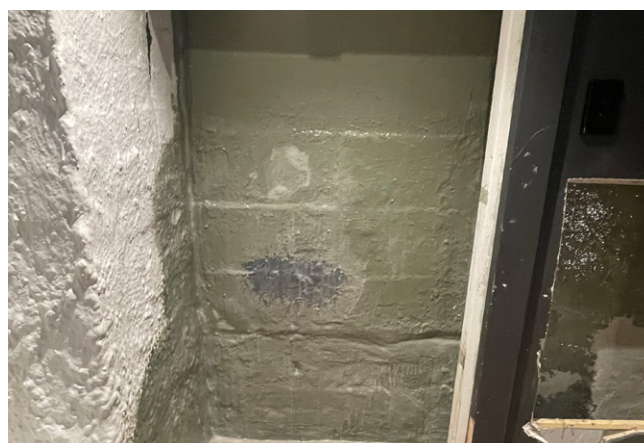
Pic 1. The basement presented multiple points of water ingress and limited available working space.
