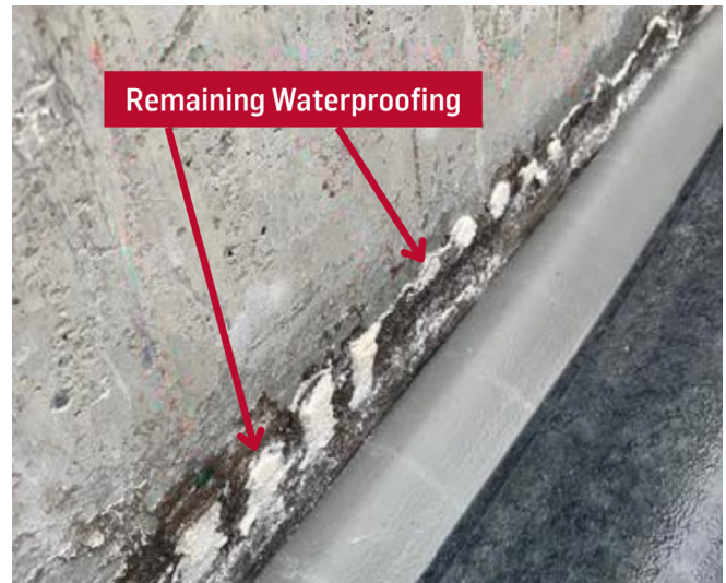
Pic 3. Remaining waterproofing and adhesive residue can be seen on the exposed substrate.
