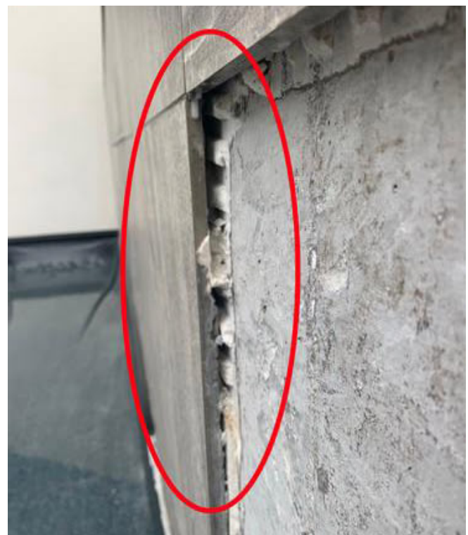
Pic 2. Tile separation from the substrate is visible.
