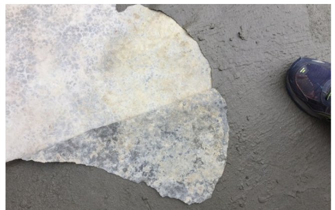
2. Delamination of membrane from substrate
