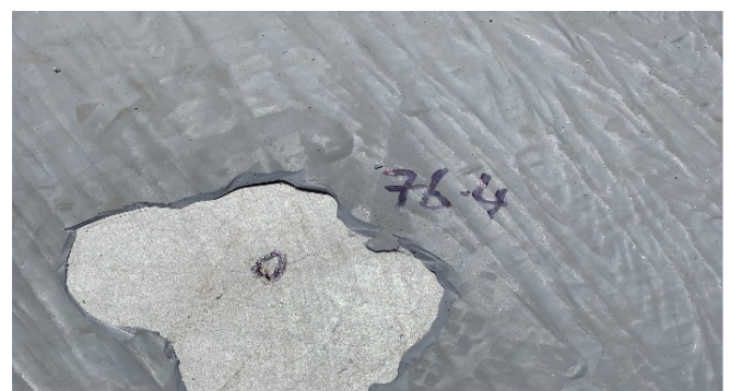
3. Delamination of membrane, high moisture content
