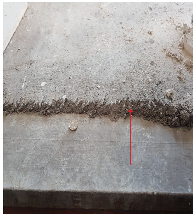
Pic 1. Crumbly Screed, incorrect MPA. Refer to Pic 1 and 2
